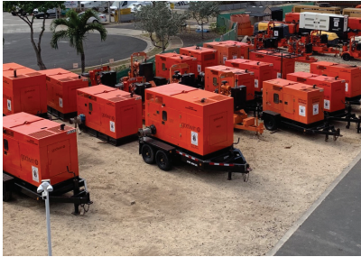
Dri-Prime Pumps for Sewer Bypassing & Dewatering
